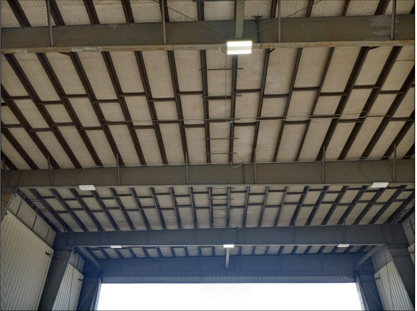
Above: Site photograph depicting typical hangar bird netting & high bay light fixtures.
