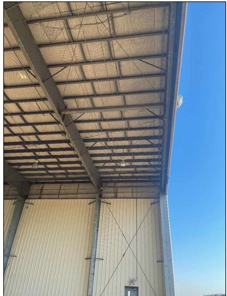
Below: Site photograph depicting damaged bird netting.
